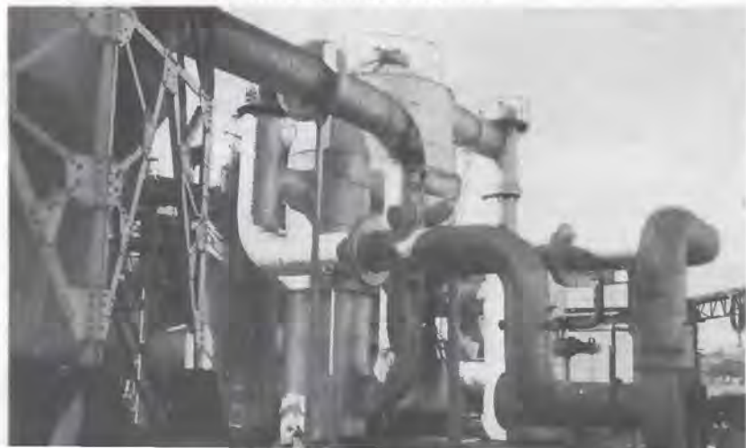
The sulphuric acid plant.
