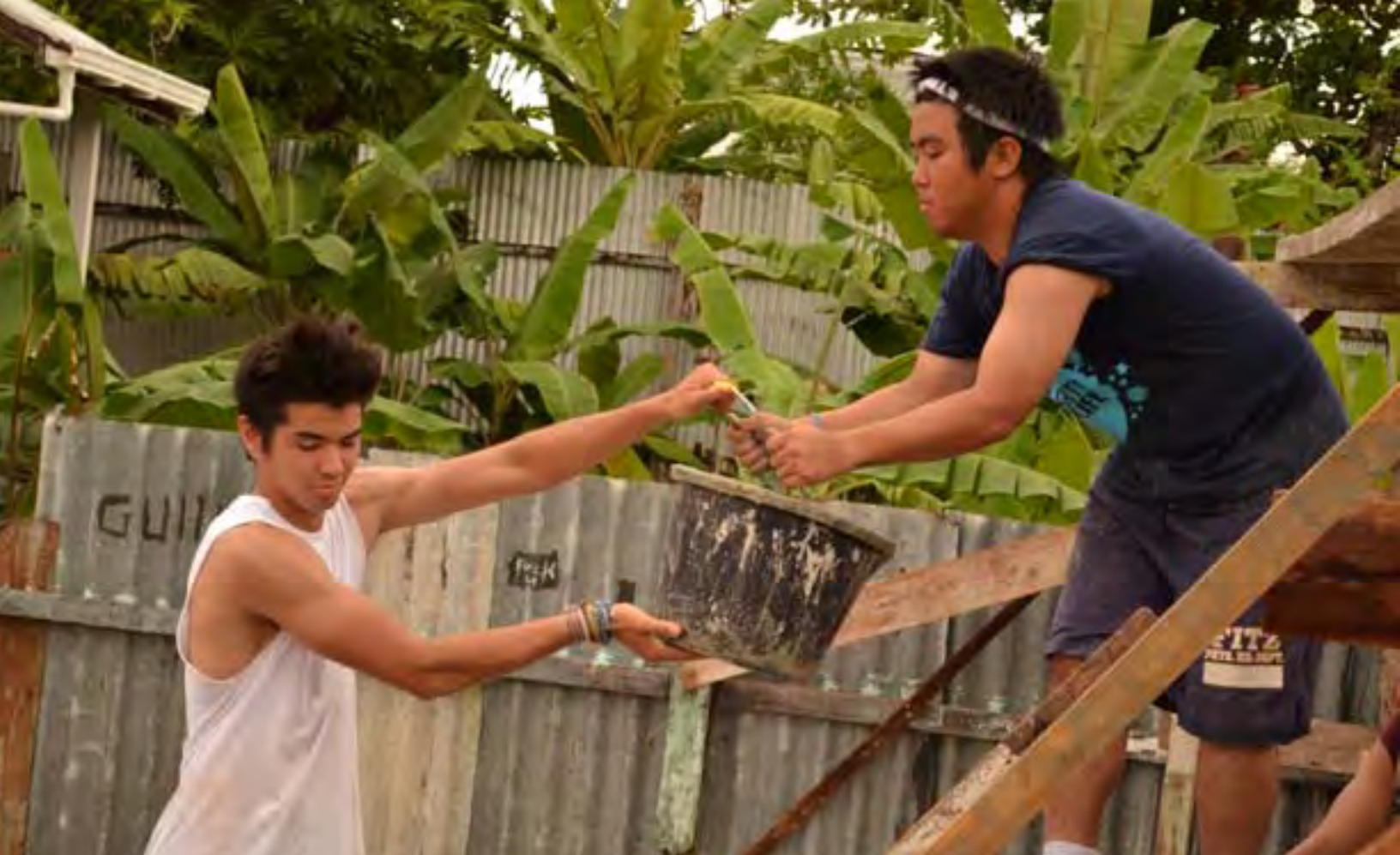
Above: Josh Hunter and Masahiro Abe help mix cement on-site at a house building project in Guyana
